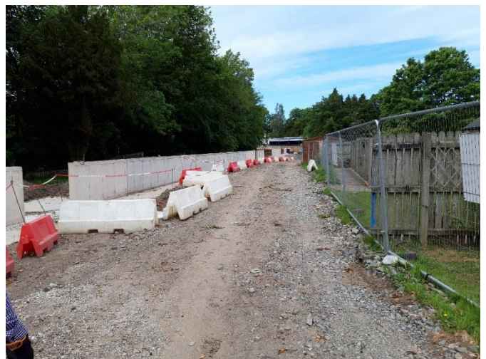
Above: Flood wall to the rear of Rickerby Court properties
