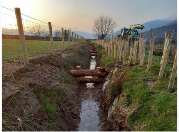
Photo 3 - Another photo of restored hedge and leaky dams above Keswick. Image: West Cumbria Rivers Trust
