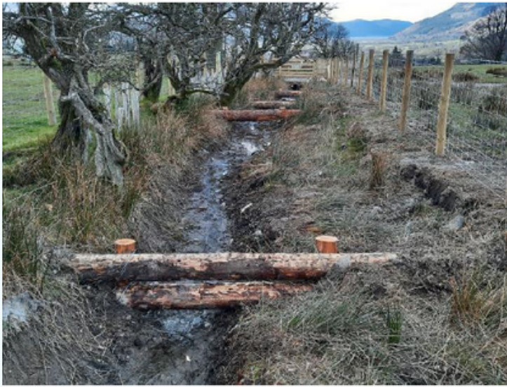
Photo 2 - Leaky dams and hedge restoration in ditch flowing directly down into Keswick. Image: West Cumbria Rivers Trust
