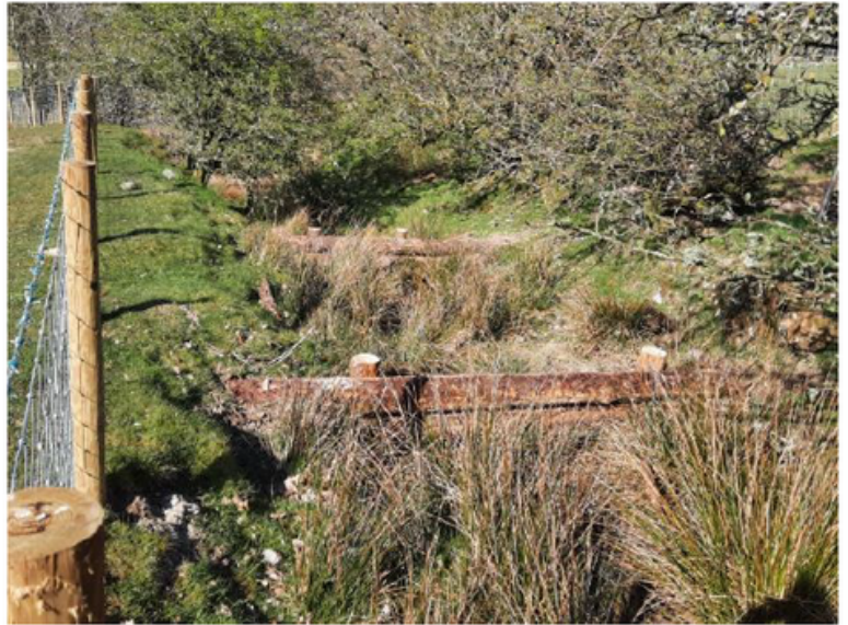
Photo 1 -Leaky dams in 2m wide ditch above main A591, flowing into Keswick.
