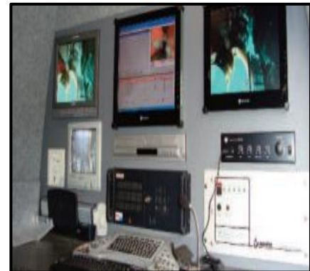
Inside a CCTV vehicle
