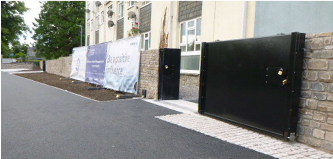
Figure 8 - Photograph of a flood gate in the open position, installed in the Waterside area of Kendal
