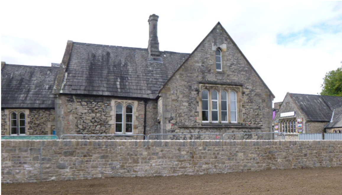
Figure 6 - Completed section of stone clad EA flood defence wall at Nether Hall, Kendal
