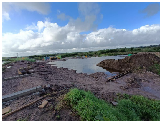
August Bank Holiday overtopping 23 – water directed into spillway area
