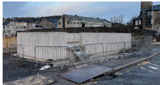
Motor Control Centre Building
