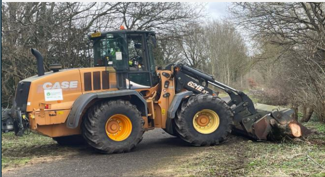
Tree blockage clearance on Micker Brook in Cheadle
