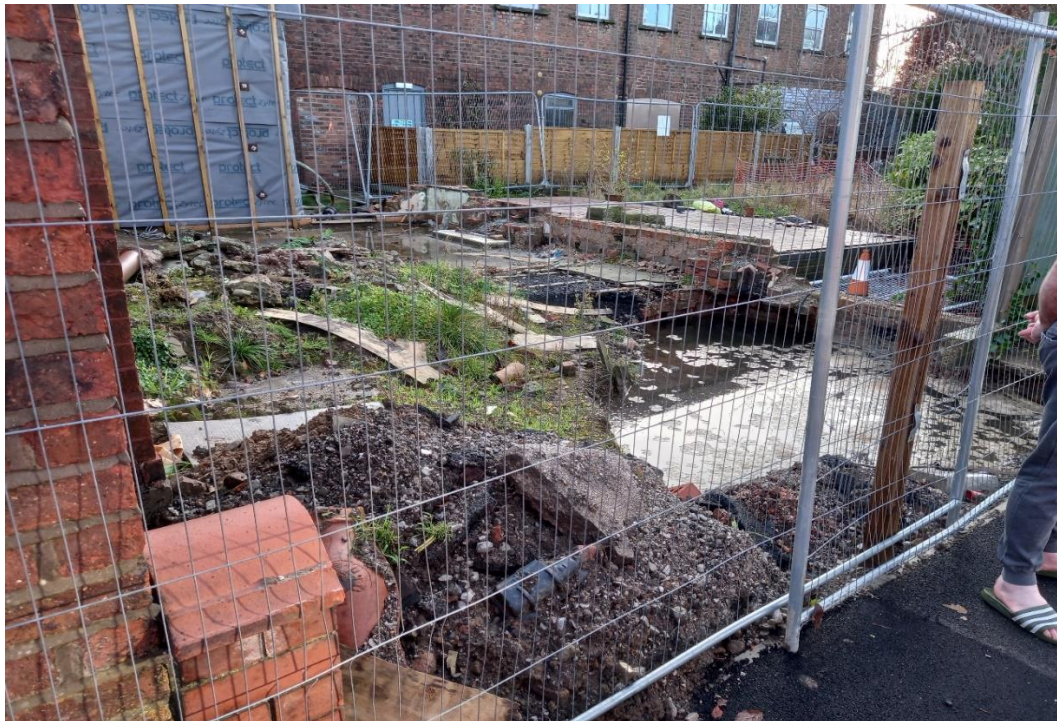
Figure 2: Site where 18 Hobson Street was previously demolished. Sink hole (open section of culvert) to the right of the photo demonstrating water levels near ground level during a dry day (not raining) and not flowing freely downstream.
