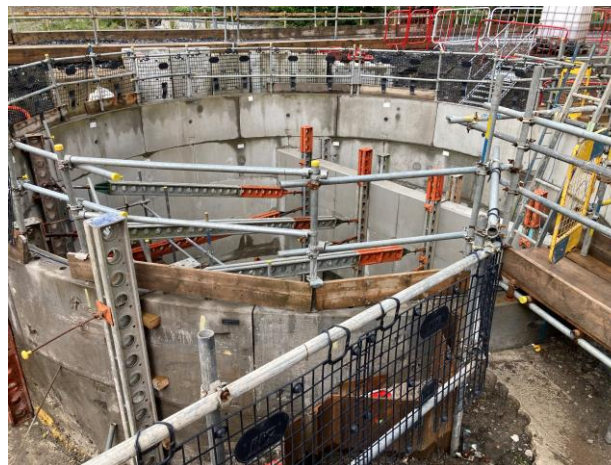
Wet Well Shaft – Underground housing of the pumps for Stock Beck
