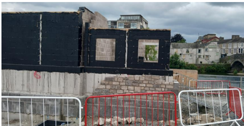
Motor Control Centre Building – Housing for all the electrical equipment for the Stock Beck pumps
