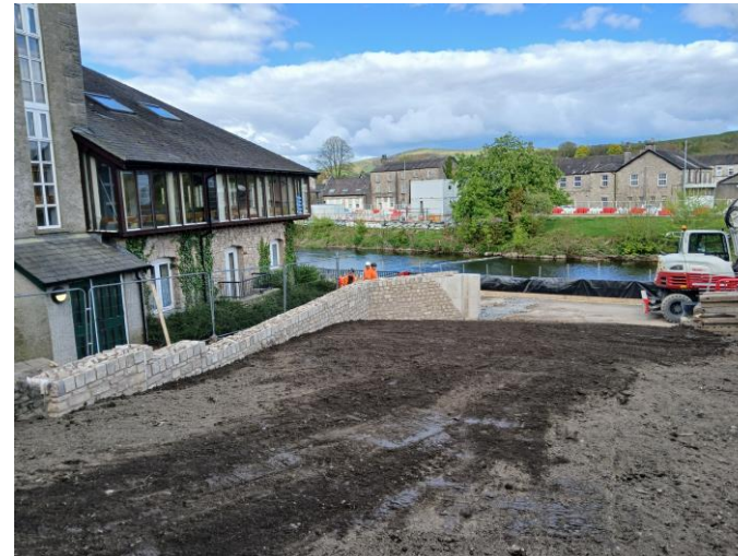
Waterside Flood gate
