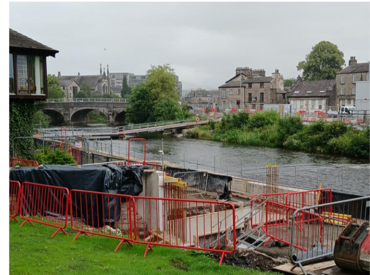
Waterside Flood gate
