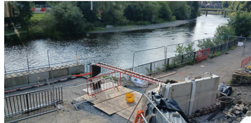
Waterside Flood gate
