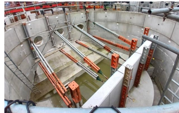
Wet Well Shaft – Underground housing of the pumps for Stock Beck
