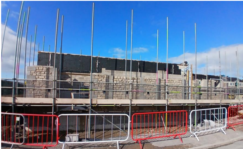
Motor Control Centre Building – Housing for all the electrical equipment for the Stock Beck pumps
