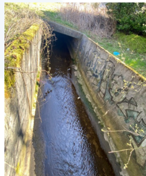
Image: The Flood Hub - Culvert
