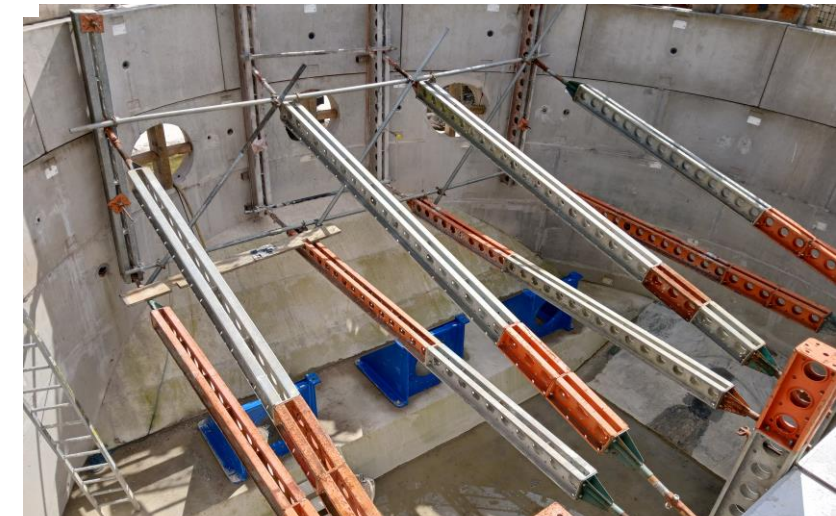
Wet Well Shaft – Underground housing of the pumps for Stock Beck
