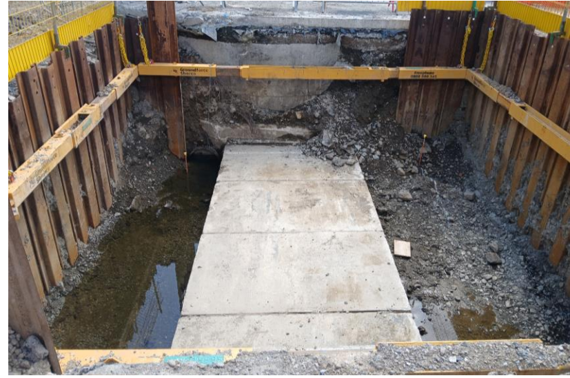
Sewer Diversion – Sheet piled area for the underpass chamber once Stock beck culvert is removed
