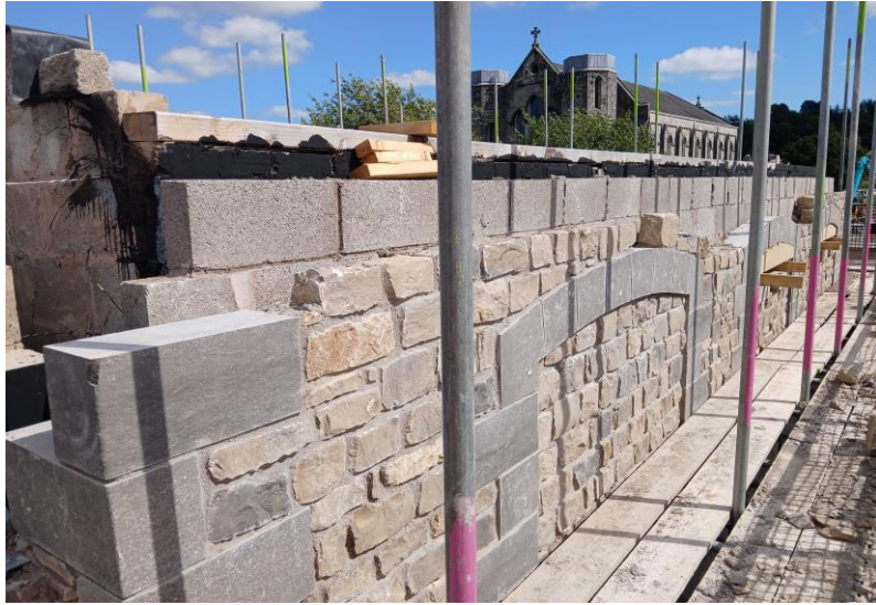
Motor Control Centre Building – Housing for all the electrical equipment for the Stock Beck pumps
