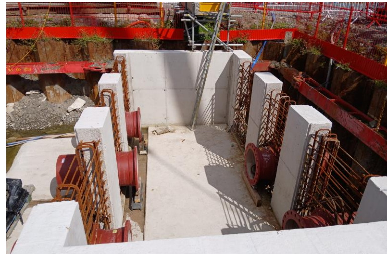
Valve chamber – Holding the pipe valves that pump Stock Beck onwards to the outfall
