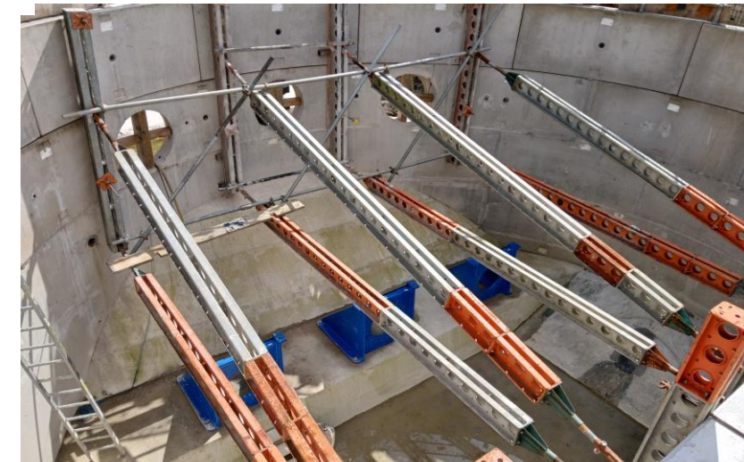
Wet Well Shaft – Underground housing of the 3 pumps for Stock Beck
