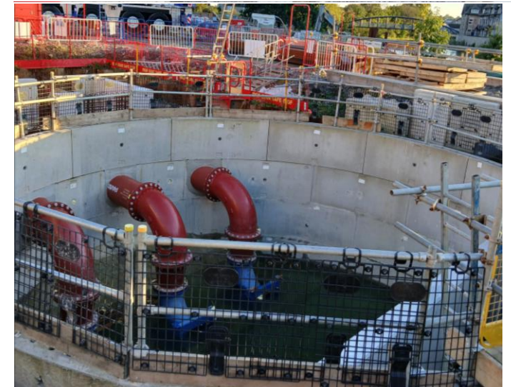
Wet Well Shaft – Underground housing of the 3 pumps for Stock Beck
