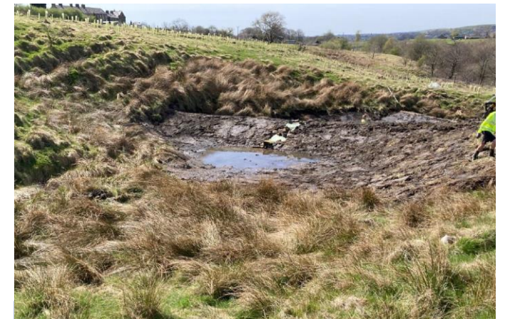
Previous NFM works which passes normal and low flows, but attenuates peak flows during storms.
