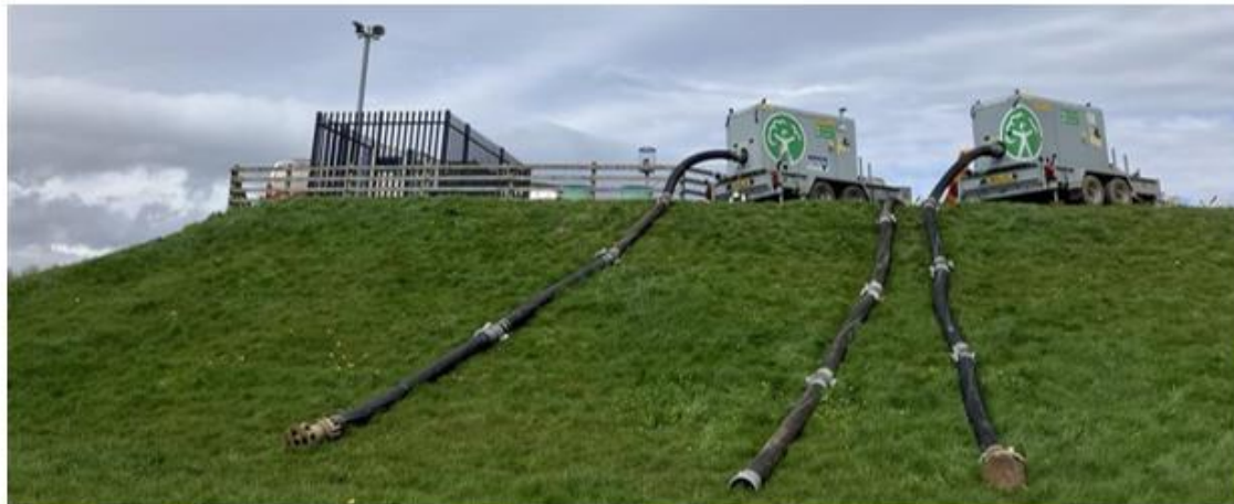
Contingency Plan Testing and Training – Durranshill Pumping Station, Carlisle
