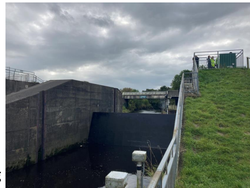
Garstang Flood Storage Basin Control Gate testing and training
