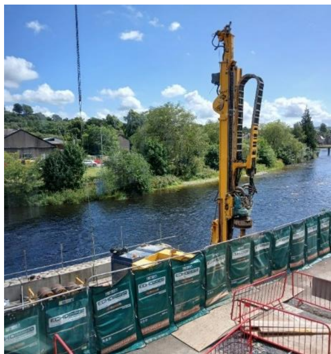
The piling rig which will be used and located on the temporary riverside platform
