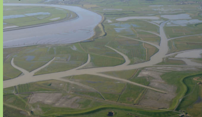
Image: The Environment Agency. Hesketh Out Marsh West in the Ribble Estuary during the construction phase
