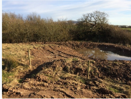
Images: West Cumbria Rivers Trust. Scrape, photo on right shows channel diverting water from field.
