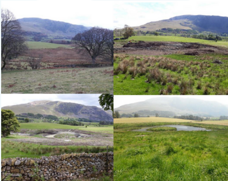
Photos 1 - 4 showing the field before the works, during the works and afterwards. Images: West Cumbria Rivers Trust
