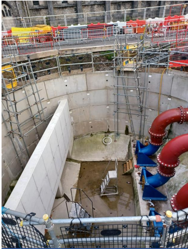
Wet well – Stock beck will be pumped from this area in flood conditions
