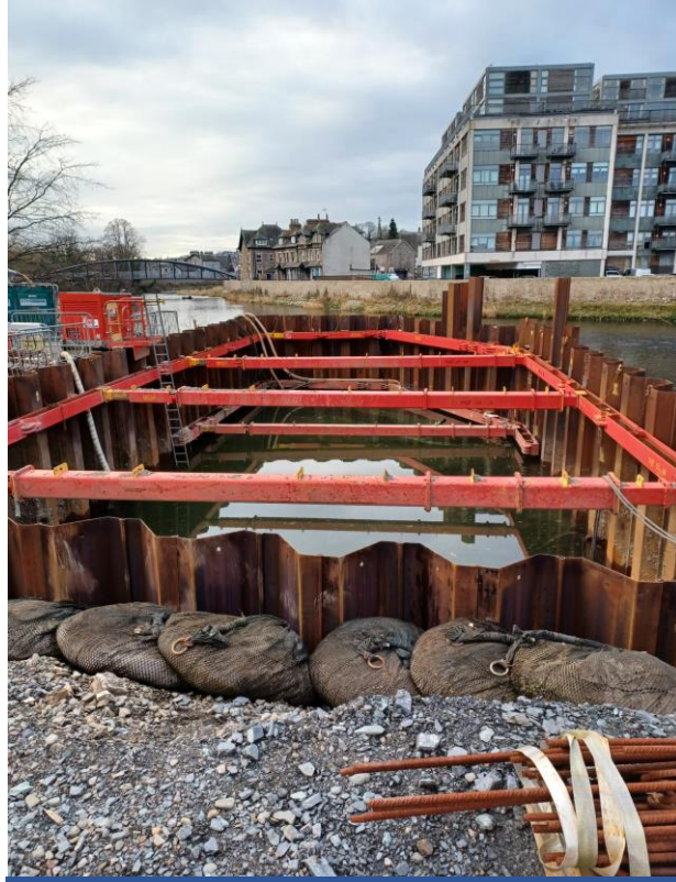
Cofferdam – Area requiring pumping due to ground water entering the excavated area
