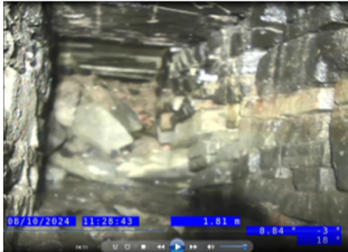
Figure 3 (left): CCTV from new 1.5m chamber looking downstream from Ryle Street towards Park Lane – shows blockage remaining beneath no. 19 Ryle Street.
