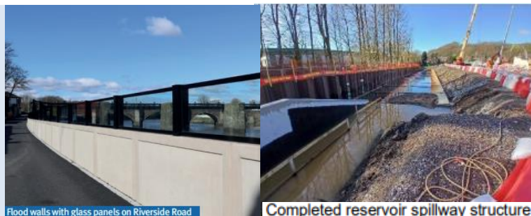
Flood walls with glass panels on Riverside Road
