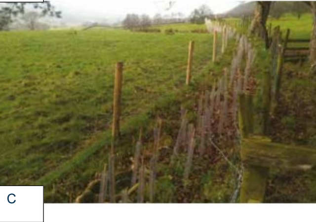
Figure 9. Bunds (A and B) and kested hedge 41 being constructed across primary flow pathway.
