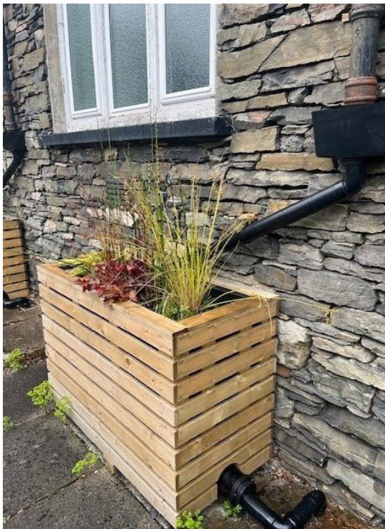
Downspout SuDS planter
