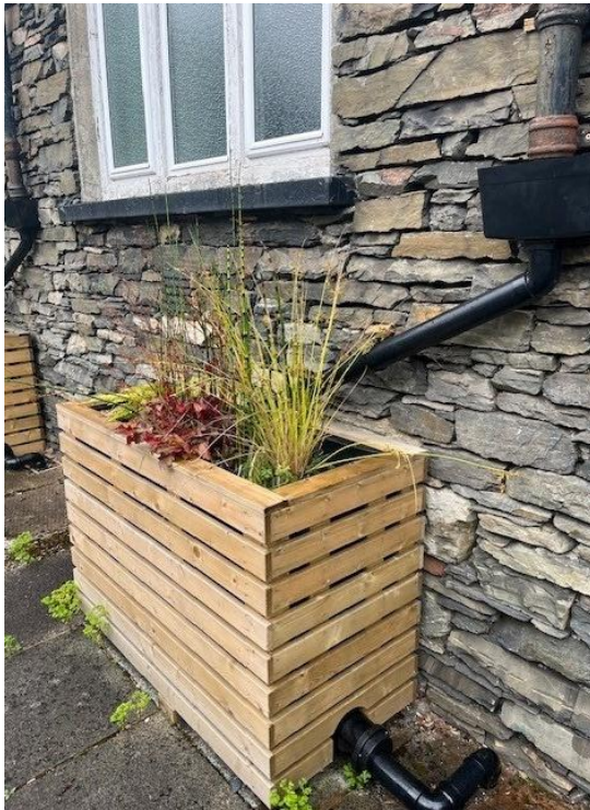
Downspout SuDS planter
